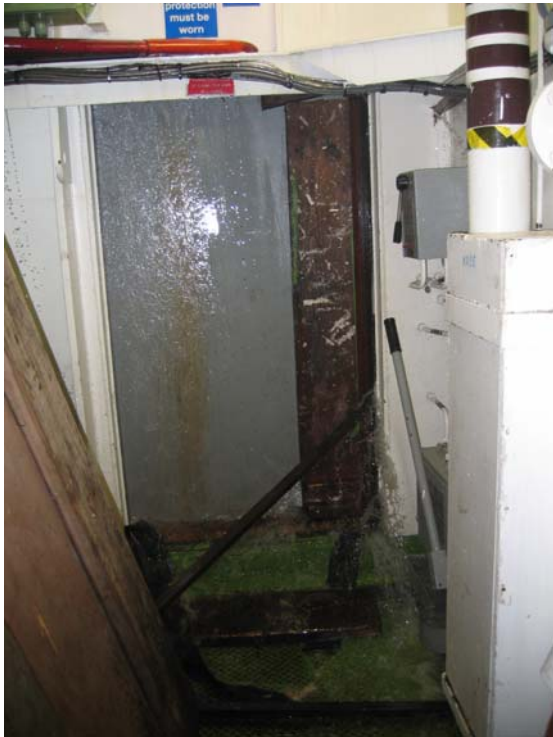
Figure SMO.2 Damage control measures in the engine room after the flooding.
